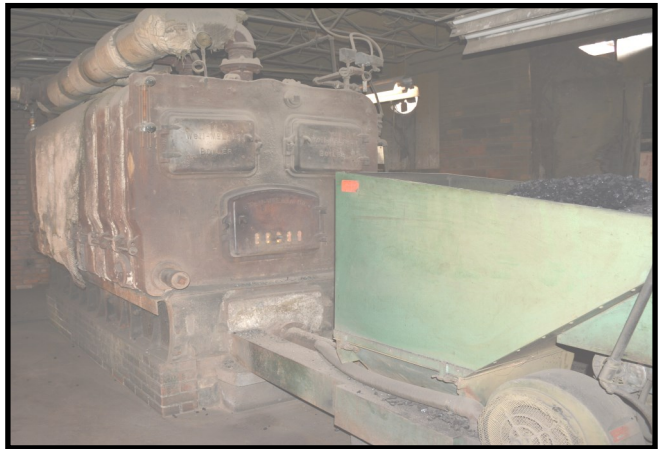
This original coal burning furnace has been in our family for 71 years, ever since the school was built in 1945. It heats the old part of the school, including the gymnasium.
